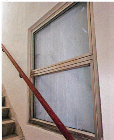
Photo 1(d): Staircase Window (Photo taken after the fire)
