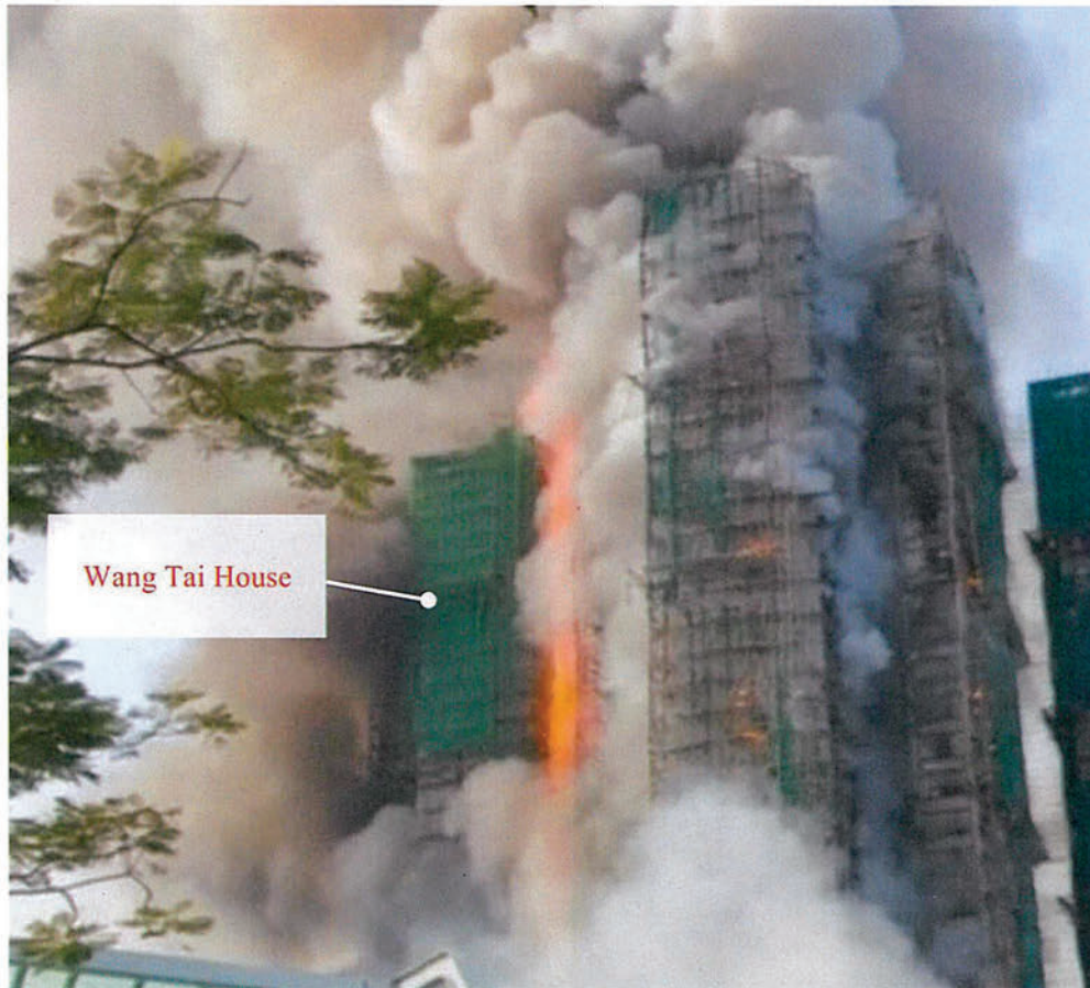
Photo 7: Rapid Vertical Fire Spread along the East Re-entrant of Wang Tai House at 1516 hours
