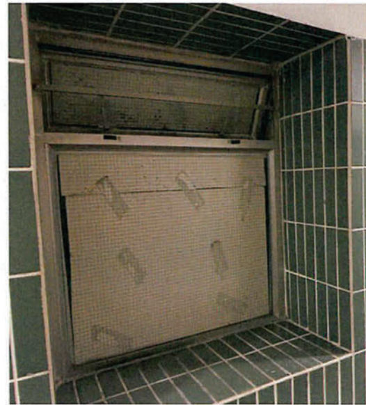
Photo 1(b): Lift Lobby Window (Photo taken after the fire)
