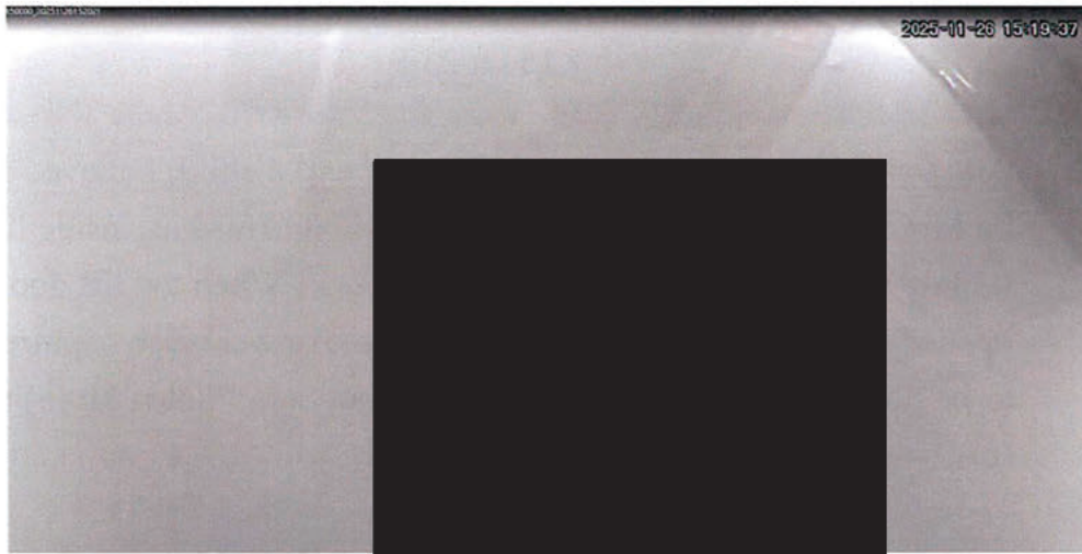
Photos 10 (a) to (c): CCTV Screenshots Showing Internal Condition of Lift L13 on 24/F
