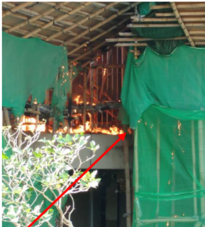
Initiation of fire at Flat roof of Re-entrant of Block F 14:50 | 26 Nov 2025
