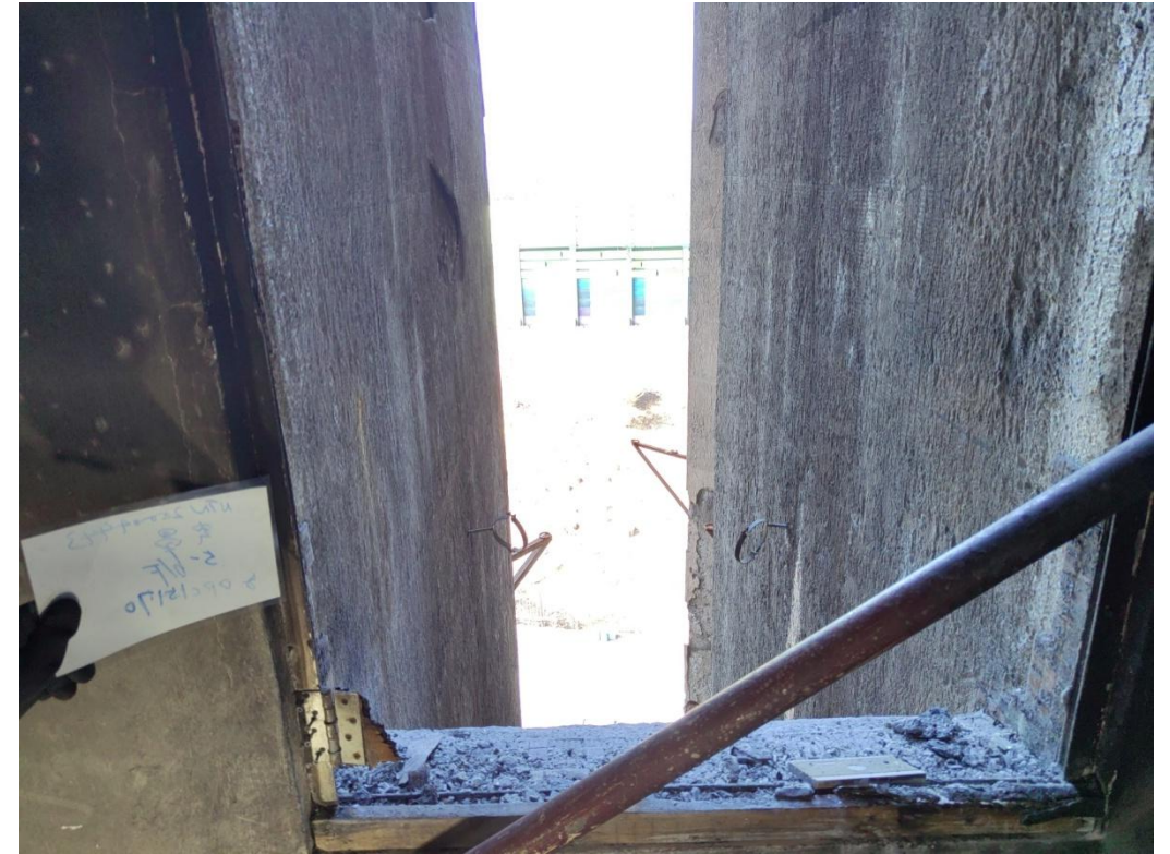
Replaced temporary wooden door burnt out
