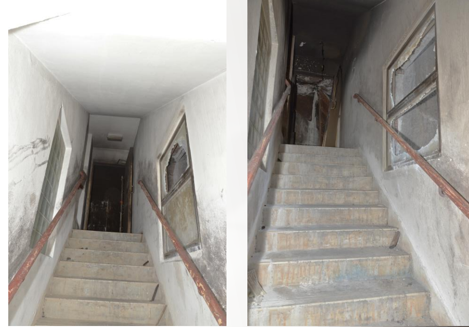
Wang Cheong House S/C Windows Broken by FS personnel
