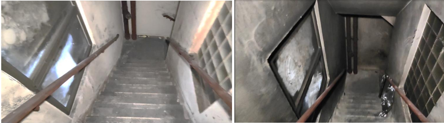
Wang Cheong House S/C Windows Remained Intact
