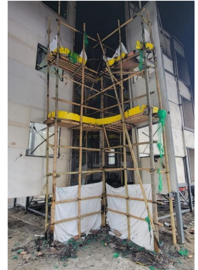
Post-Fire Condition in Test 12 using Safety Nets collected Wang Chi and FR Canvas
