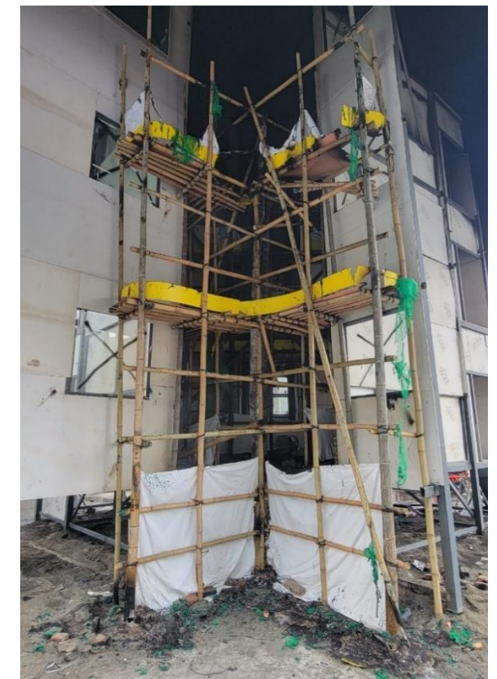
Post-Fire Condition in Test 12 using Safety Nets collected Wang Chi House and FR Canvas
