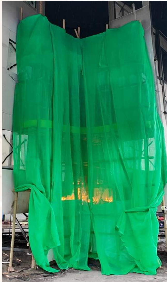
No Fire Spread along Safety Nets in Test 11
