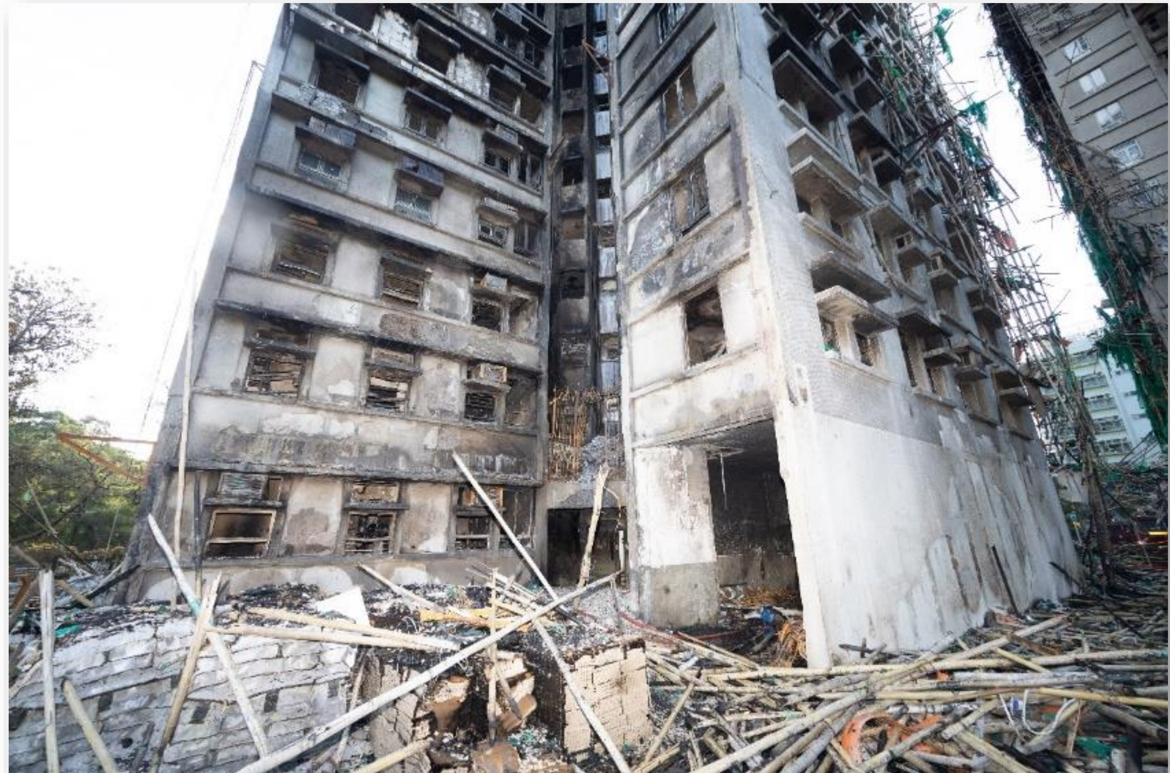
Post-Fire Condition Outside East Re-entrant of Wang Cheong House
