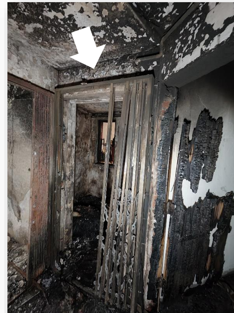
Damaged Unit Entrance Door
