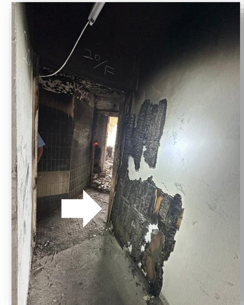
Damaged Smoke Stop Door
