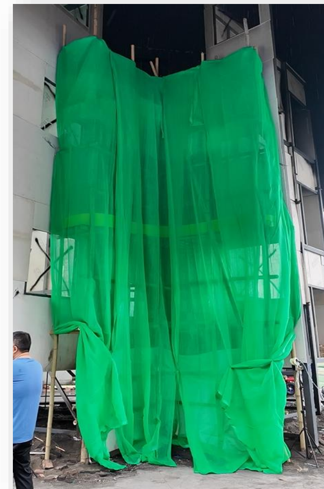
Post-Fire Condition in Test 11 using FR Safety Nets and FR Canvas
