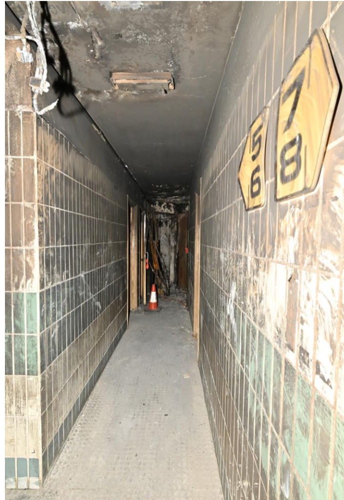
View of corridor from Flat 107-108 towards Flat 105-106, with close-up view at Photo A (more severe heat damage at the end of Flat 105-106)
