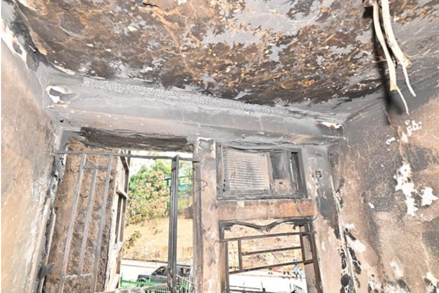
View of living room window (more severe spalling on the concrete window overhang outside rendering it an irregular surface)
