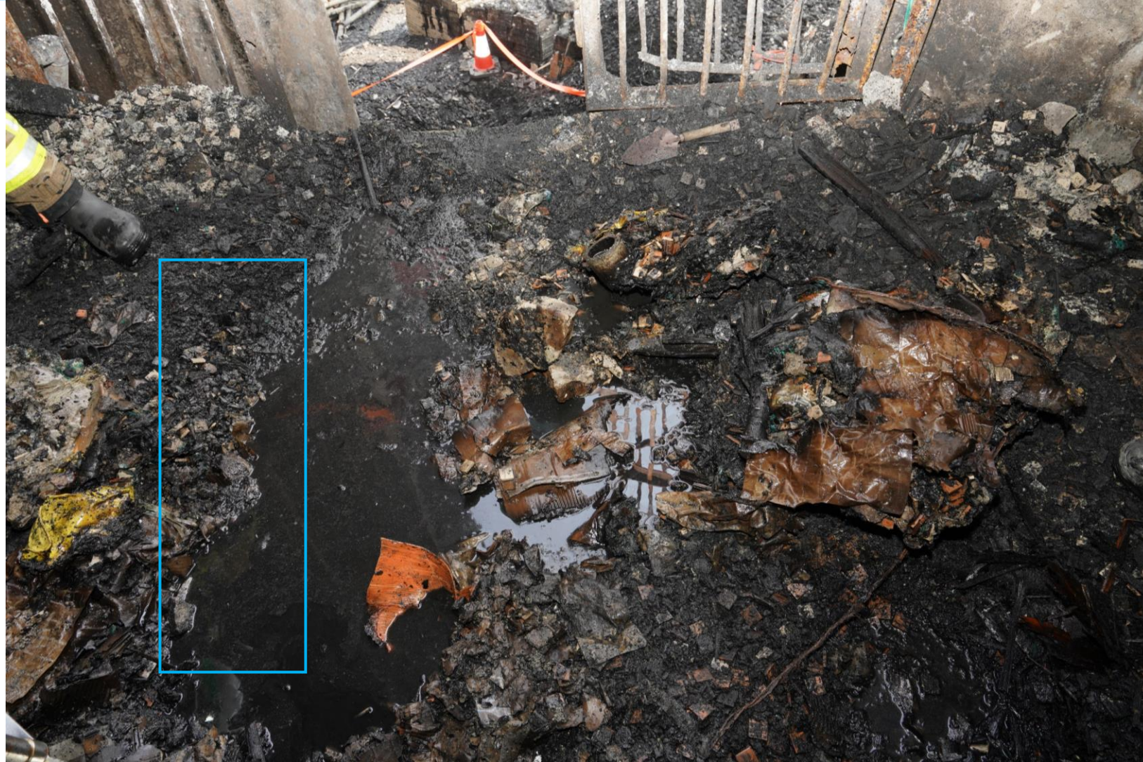
Photo 26: View of seat of fire toward the metal gate (substantial amount of burnt remnants of carton paper boxes, found in the area next to the metal fence near Flat 105). Foam board fragments and a corrugated plastic board ( A ) and a woven plastic bag of backing papers ( B ) were recovered in the middle area as marked in the blue rectangle
