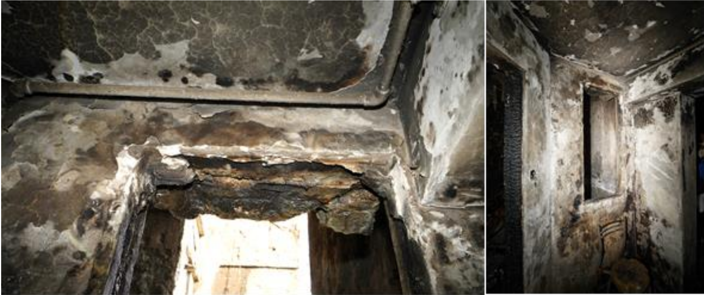
View of entryway window (more severe spalling on the concrete window overhang than the inner wall)
