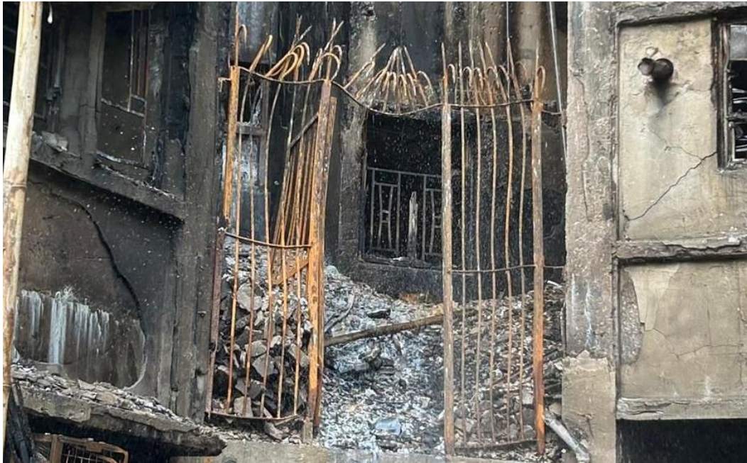
Photo 6-1: Debris Piled up on the Flat Roof outside Flats 104 and 105
