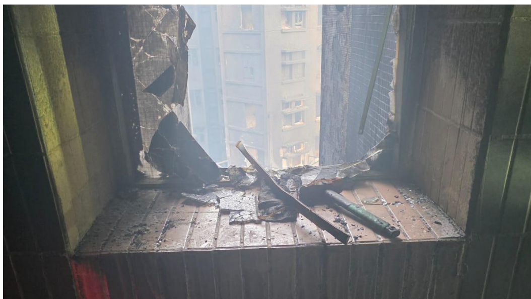
Photo 7-10: Photo Showing the Window Sill on the 31/F
