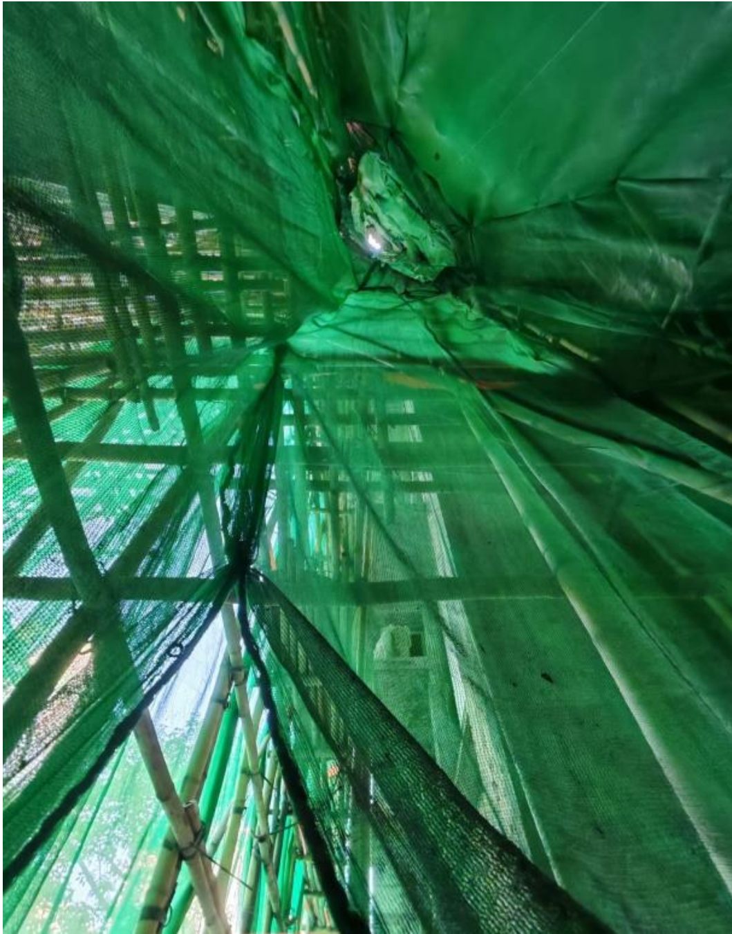
Photo 4-13: Triangular Channel Leading from Flat Roof to R/F at the Re-entrant
