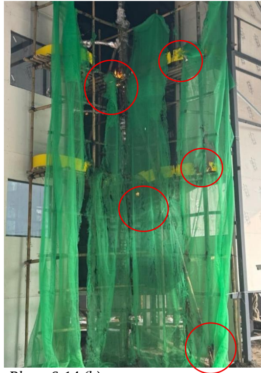
Photo 6-14 (b): Fire Spread along Non-FR Safety Net
