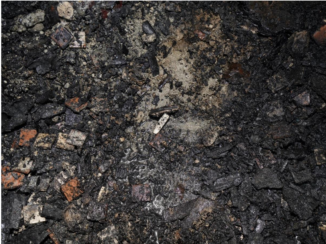
Photo 6-3: One of the Cigarette Ends Found at the Subject Flat Roof
