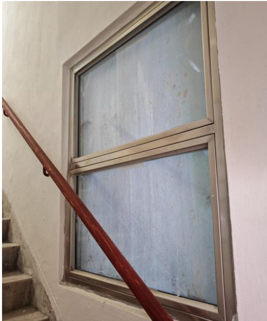
Photo 4-3(b): Staircase Window (Photo taken after the fire)
