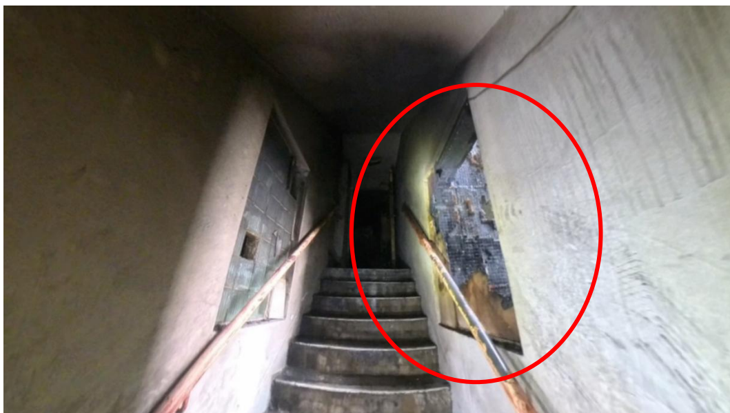
Photo 8-2: Windows Replaced by Movable Boards (Damaged by Fire) at Escape Staircase of 10-11/F of Wang Tai House
