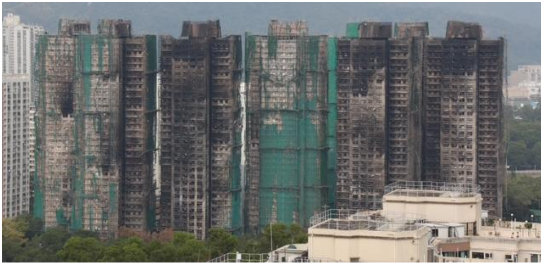
Photo 5-12: Post Fire Condition of Wang Fuk Court
