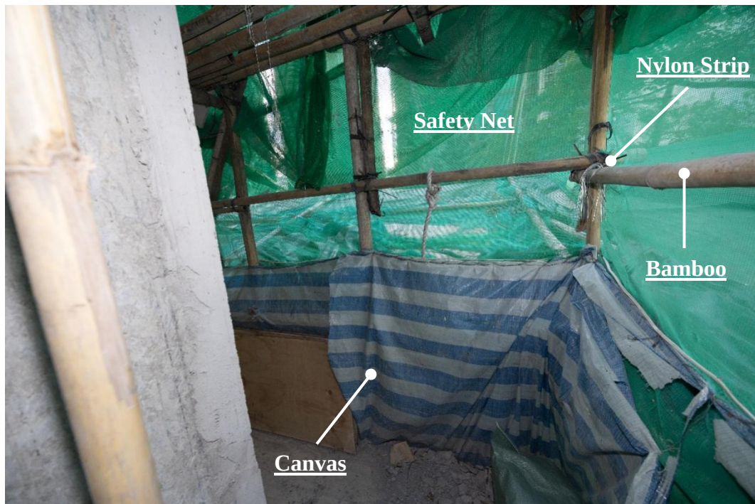
Photo 4-5: Photo Showing Different Combustibles in the Scaffolding (Bamboos, Safety nets, Canvas and Nylon strips)
