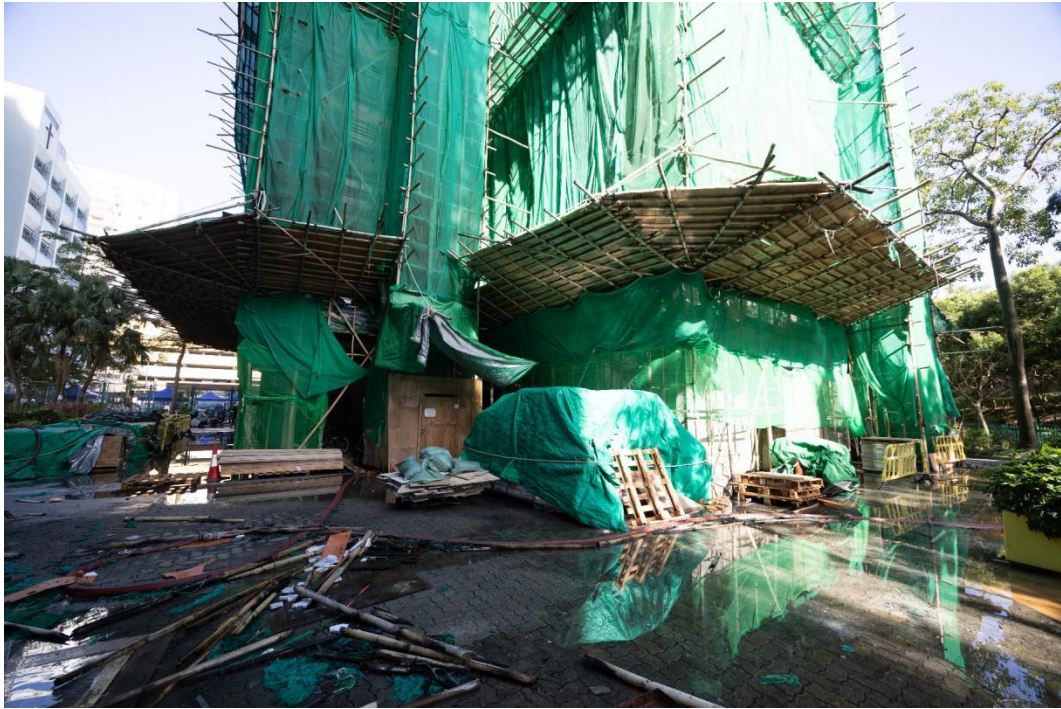
Photo 4-10: Combustible Materials Scattered at Ground Level around Wang Chi House
