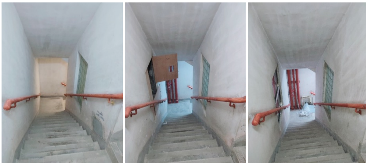
Figure 4.5. Conditions of staircases before fire
