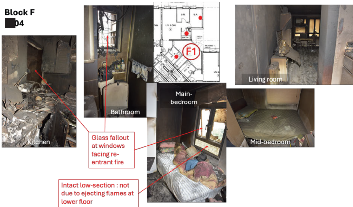
Figure 3-11. Typical unit (Block F 04) with bedroom windows exposed to re-entrant fire
