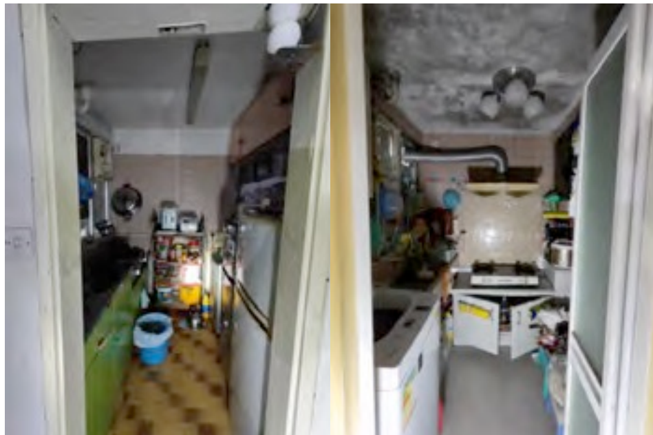
Figure 4.2. Self-closing kitchen doors replaced by non-fire rated doors
